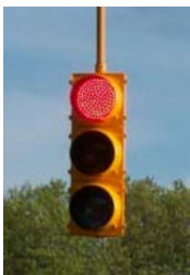
LED Traffic Signal
